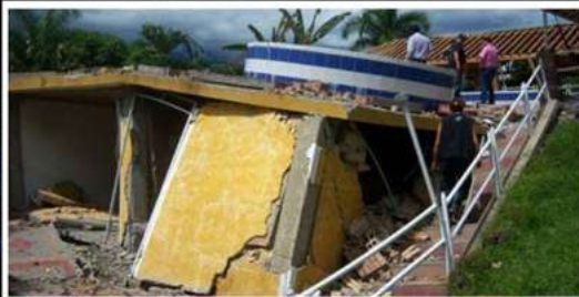
Cracks threaten village of La Mesa, Cundinamarca (Colombia)
